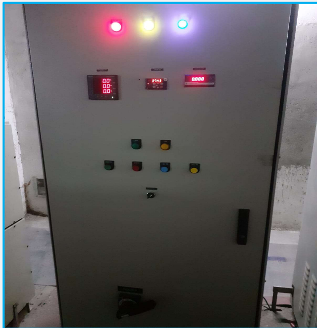
After Modification- Fly Ash unloading Compressor in VFD Mode
