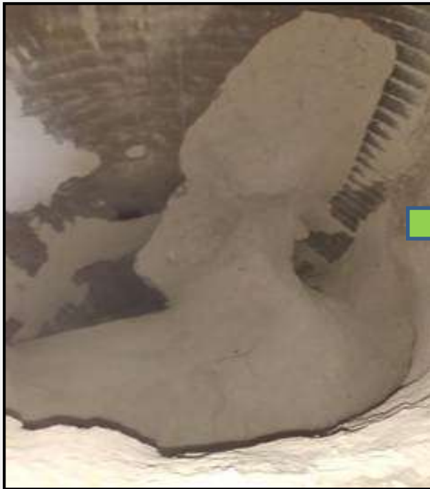
Before – Raw material hopper
