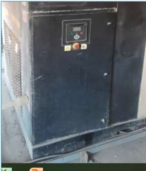
After Modification- One Compressor running
